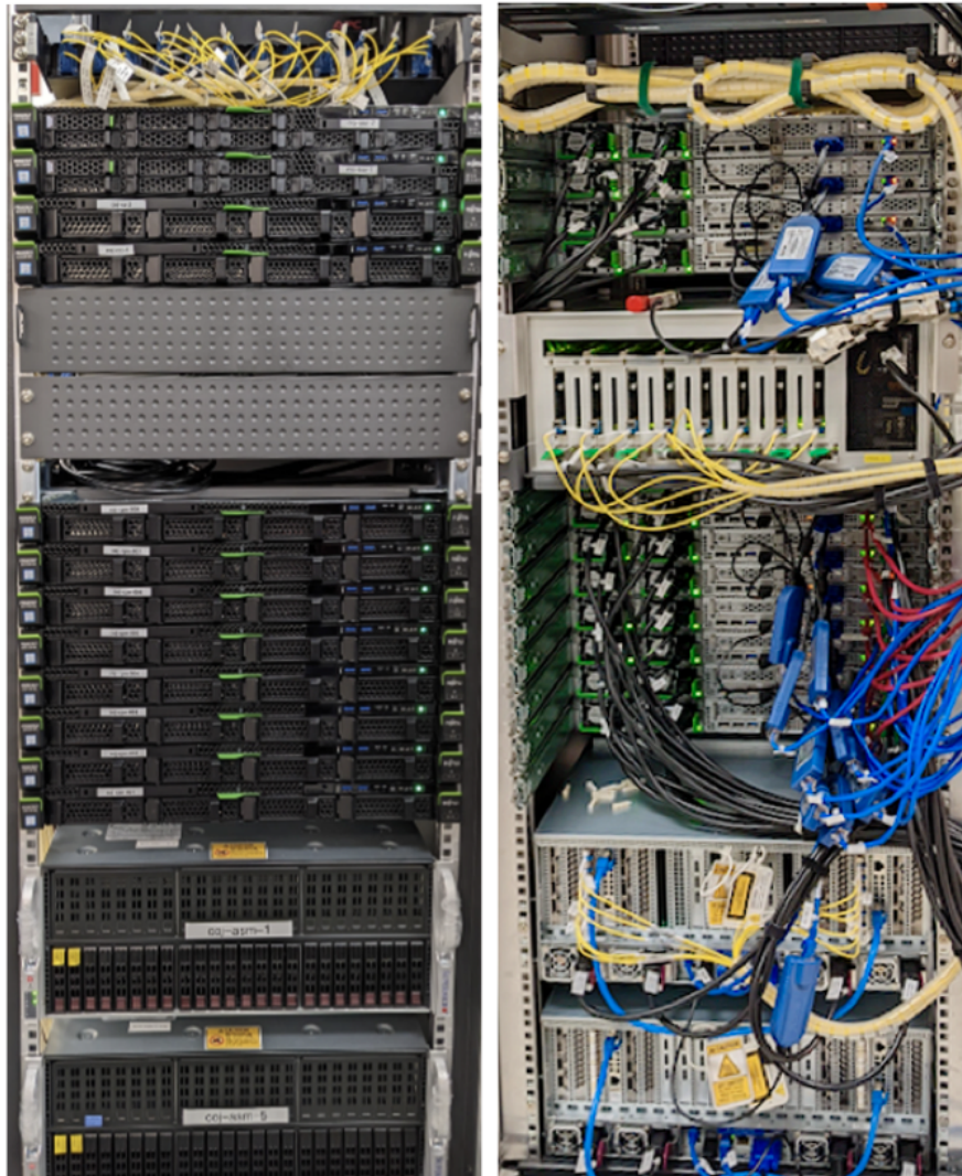
Figure 5.7: Photos of the ACA Spectrometer installed in the ACA correlator room (Credit: ALMA ESO/NAOJ/NRAO). Major components of the ACA Spectrometer were installed at four computer racks that have been used for the ACA Correlator. The photos show the front (left) and back (right) sides of the computer rack labelled “quadrant 0”, respectively. Two ASMs (one is a working server and the other is a spare server ASMs) and two ASCs (one is a working server and the other is a spare server) are installed at the bottom and upper sides of the rack, respectively. An optical splitter is installed at the most upper side of the rack. Each of the other three computer racks contains an ASM and an optical splitter.
