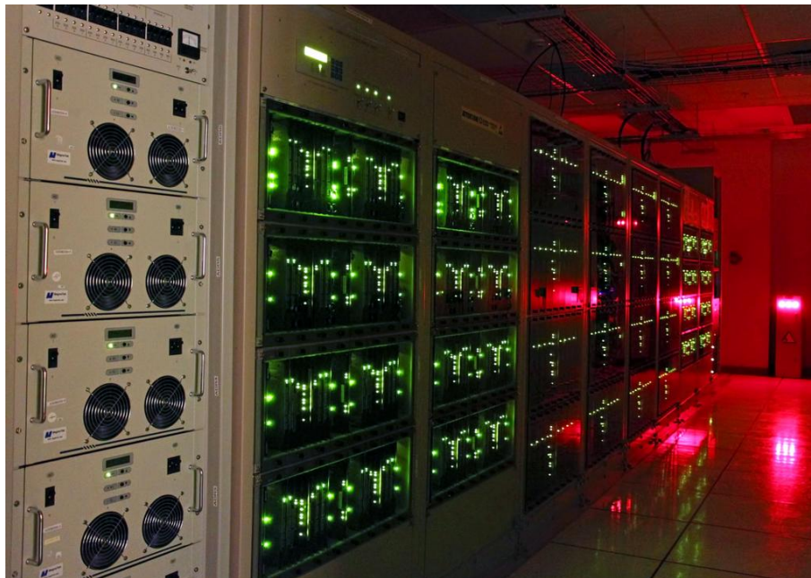
Figure 5.1: The ALMA 64-input Correlator. This view shows lights glowing on some of the racks of the correlator in the ALMA Array Operations Site Technical Building and shows one of four quadrants of the correlator. Credit: ALMA (ESO/NAOJ/NRAO), S. Argandoña
